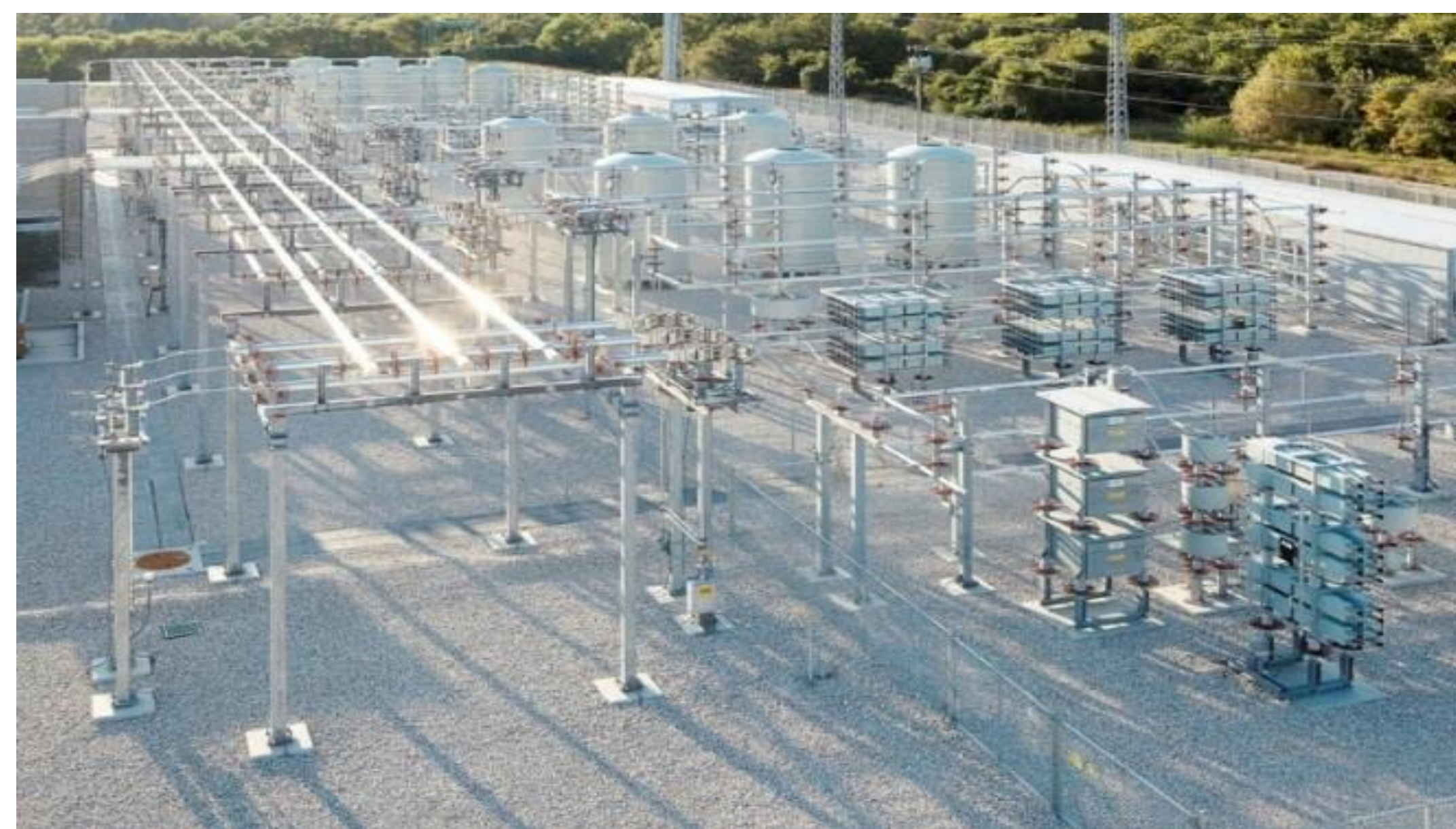
Figure 1. An ABB static var compensator outside Dallas, US. The three conductors to the left motivates the geometry considered (Fig. 3). Picture by ABB.
