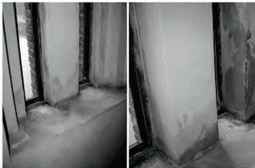
Figure 10. Observed moisture spots at the inner surface near the windows
