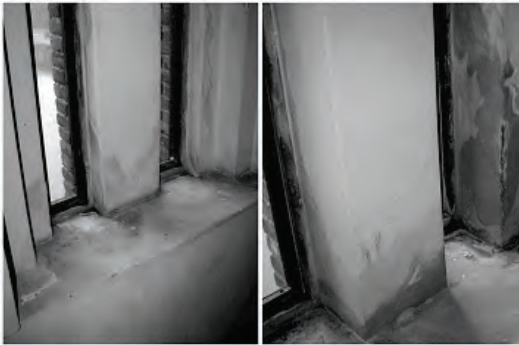
Figure 2. Observed moisture damage in the tower of the building: moist spots and efflorescence
